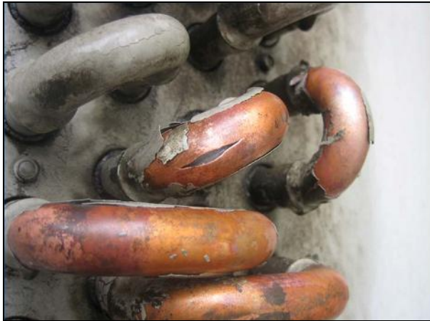
Figure 1. Typical damage in Radiator pipes as a result of freezing [1].
