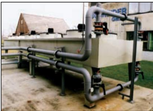
Figure 10. The dry cooler installed in the system [16]
