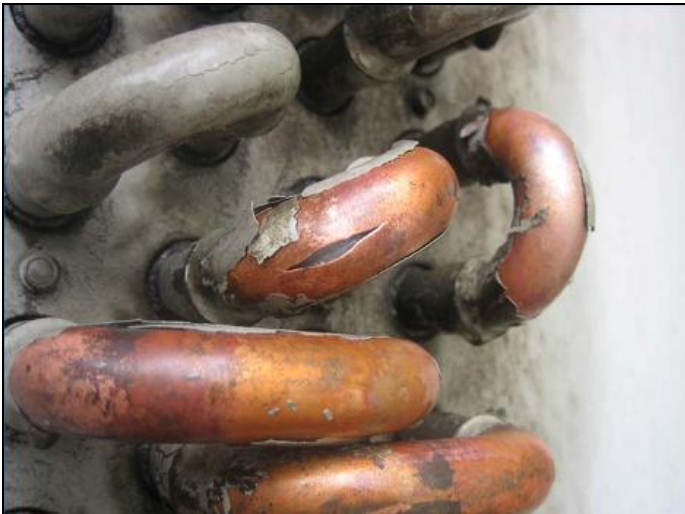
Figure 8. Typical damage in dry cooler tubes as a result of freezing [9].
